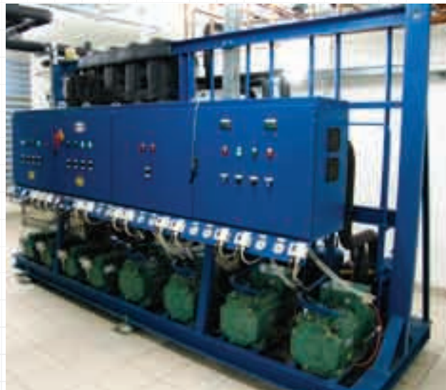
CREA compressor rack
