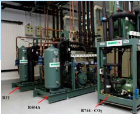
R22, R404A & R744 compressor racks
