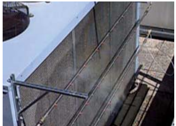
Chiller on CAREL Industries S.r.l.'s roof with 3 fans on top and water being sprayed counter-flow towards the cooling coil
